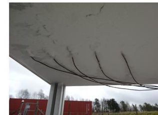
Steel plate underside after 200s release
